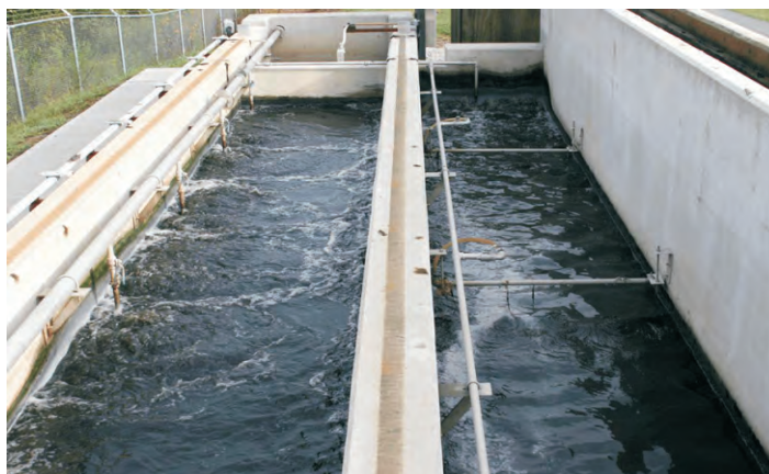
Fig 18.4: Grit and sand removal tank
